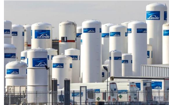
Cryogenic storage tanks
