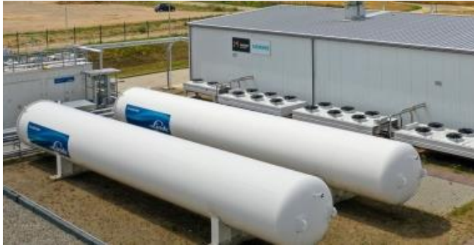
CGH2 storage Energiepark Mainz, 20-80 bar, 1000 kg
