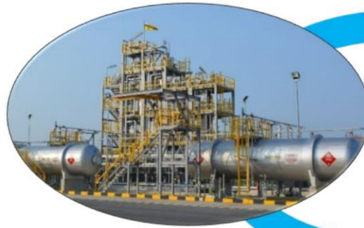
【 Brunei Hydrogen Production & Hydrogenation Plant】
