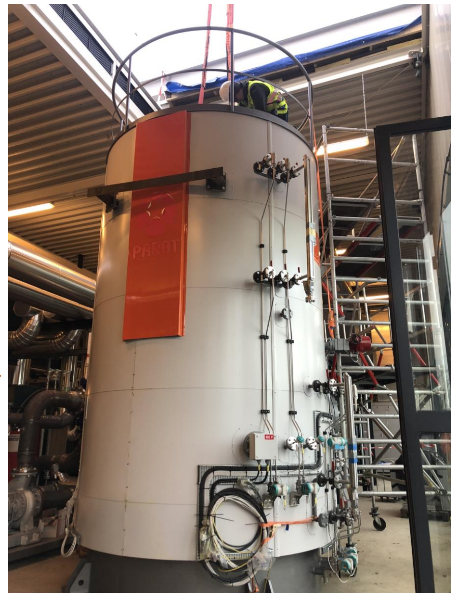
Electrode Boiler (12 MWth)
