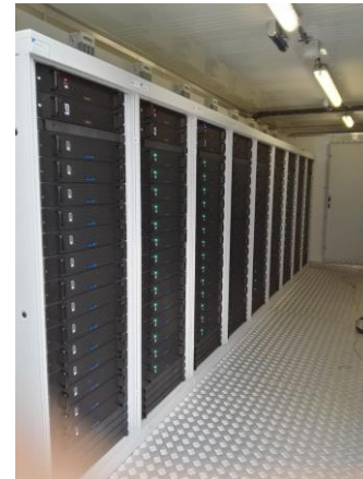
Figure 6b: SSU at project site (inside the battery cabinet)
