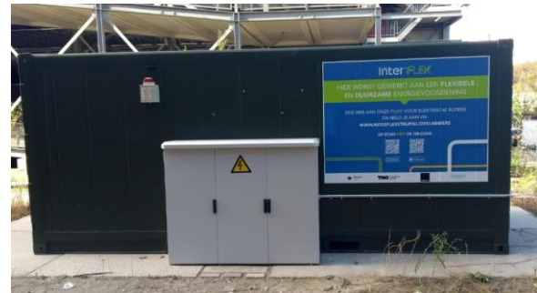
Figure 6a: SSU at project site (outside battery cabinet)
