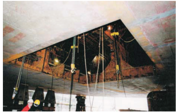
Figure 6: A large hole is bored in the underside of the 'Giant 4' to completely accommodate the conning tower of the 'Kursk'. The hole measures 32 metres by 9 metres.
