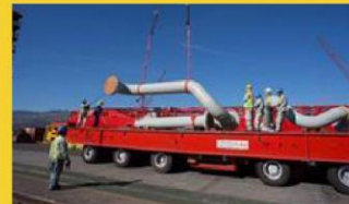
Spools to be used for the Turnaround being loaded out from Subic
