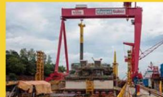
The first of the four upper tubular legs, weighing 478T, 65m long and 3.8m in diameter, was safely installed into the Depletion Compression Platform
