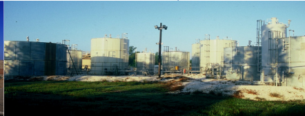
Chemical EOR, USA
