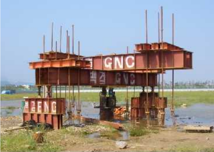
Head-down loading test on a 600 mm diameter, 54 m long cylinder pile in Busan, Korea, 2006. (Kim, Chung, and Fellenius, 2011)
