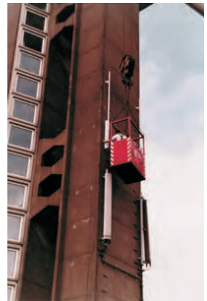
Fig. 5 Installation of one of the three sector UMTS antennas at the tower of KPN Research. The longer antennas at the bottom of the picture are GSM antennas.
