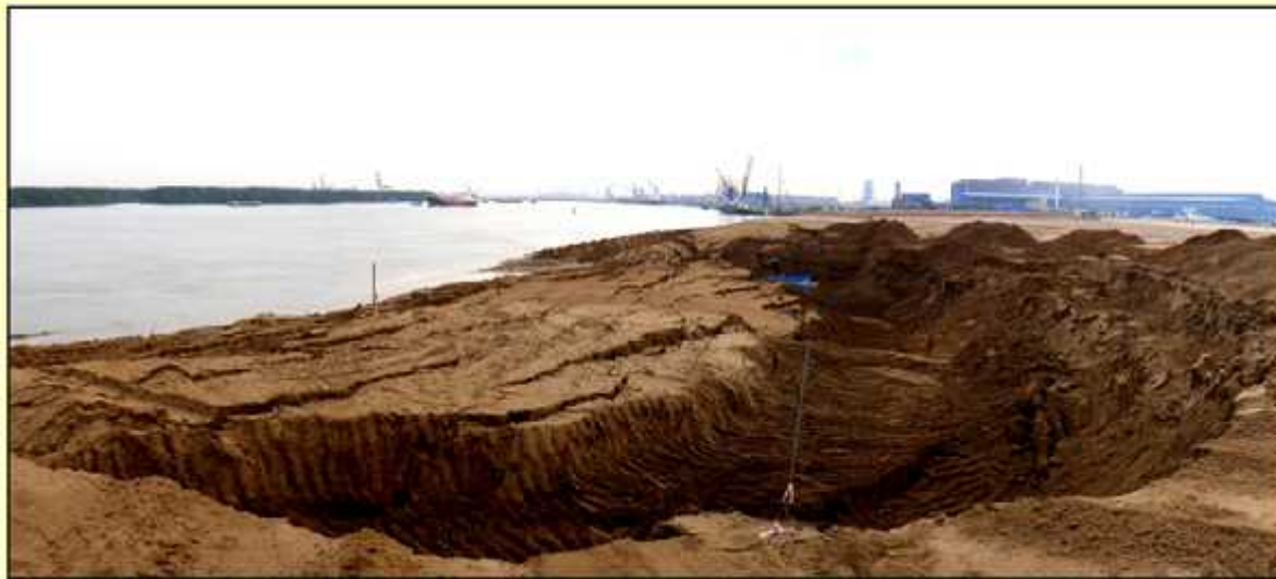
Slope failure on July 12, 2010, viewed upstream
