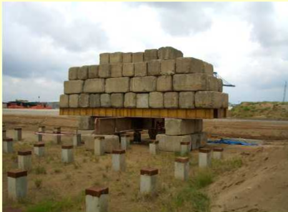
The static loading tests (CFS and CG) were carried out in September 2010, nine months after pile driving
