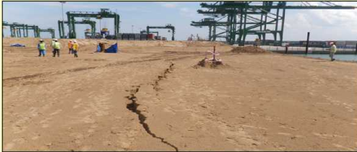
Downstream view of the first cracks that appeared at Thi Vai site along the riverbank (April 5, 2010)
