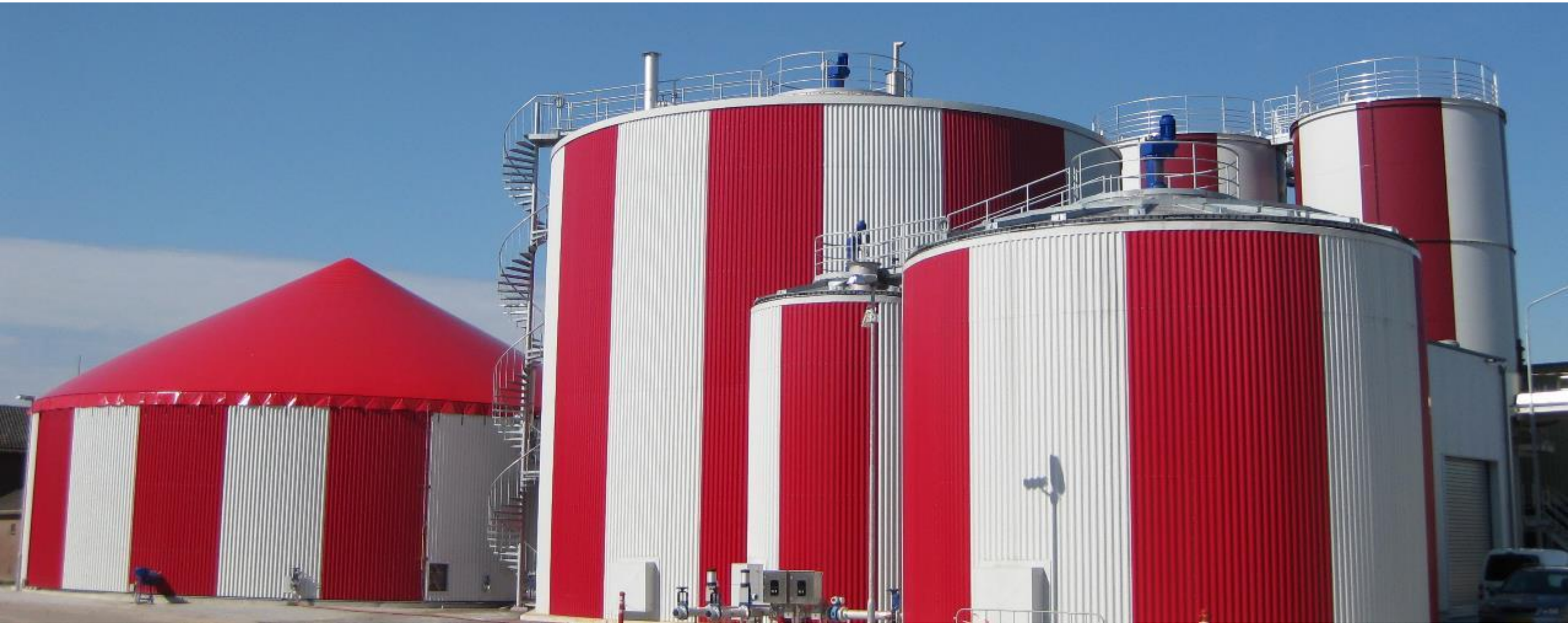
Industrial Biogas Plant Echten, Netherlands: 1,4 Mwe
