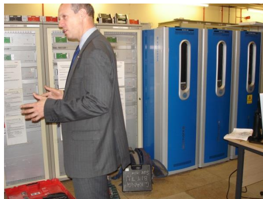
Electronic Interlocking Westrace en Westlock
