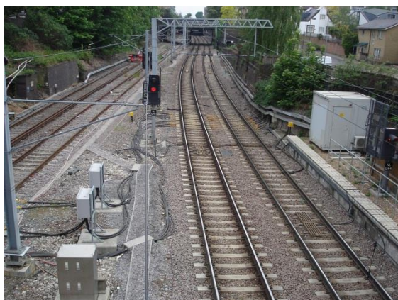
Dalston Junction 750V DC versus 25kV AC
