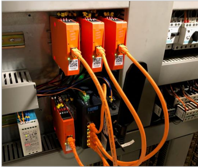
Monitoring in motor control cabinet (MCC)
