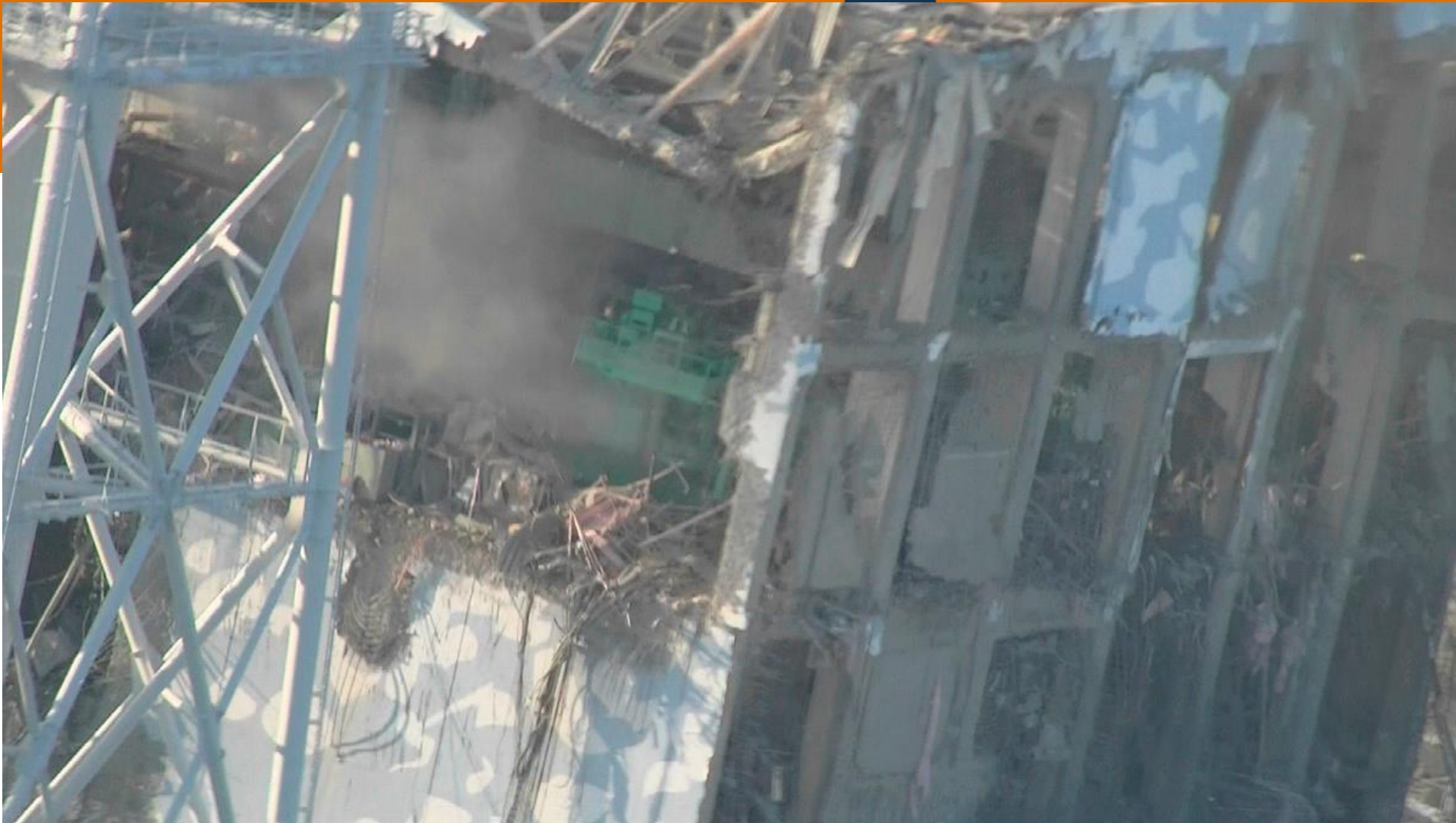
Unit 4 refueling deck (green equipment in center image is fuel handling machine)
