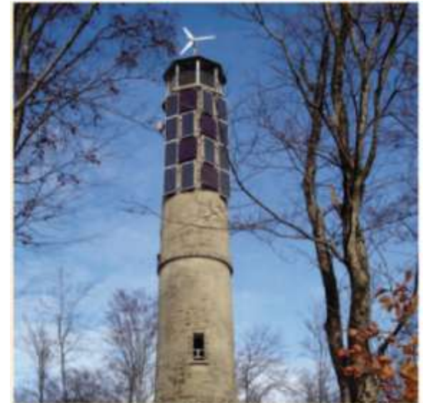
Fig. 4 The trunked radio system on the Brandeckopf tower near Offenburg, Germany, which is used for communicating with and monitoring a regional railway line, is operated with a PV hybrid system. Source: Steca Elektronik GmbH
